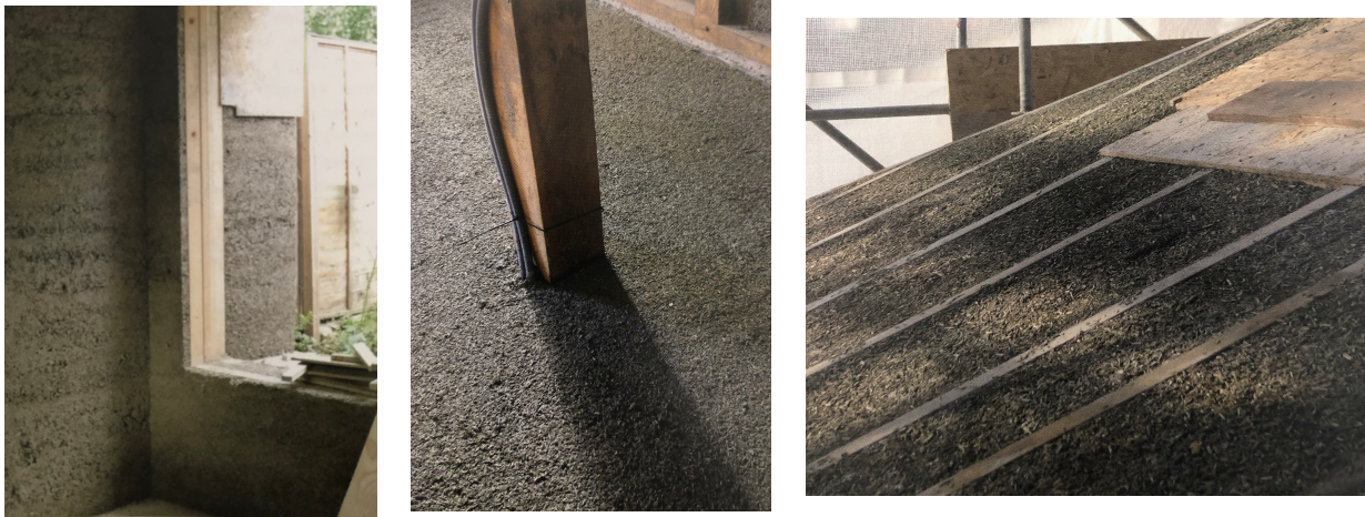
Hempcrete cast in situ in wall, floor and ceiling assemblies Source: The Hempcrete Book. Designing and building with hemp-lime
